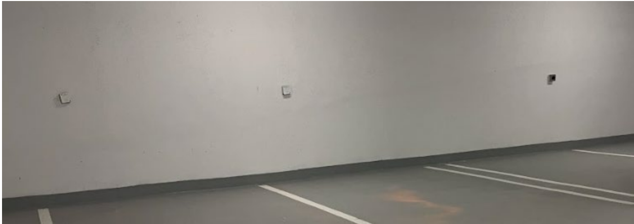
Example of EV outlets: (left two - rough in, right - active)
